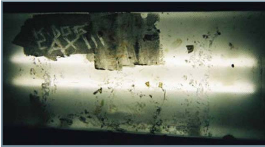
A photo of the walls from the Coke County Juvenile Justice Center Audit: A Report by the Texas Youth Commission . The report stated, "Human excrement was found floating in the [shower] drain during a September 2007 audit." Photo from TYC
